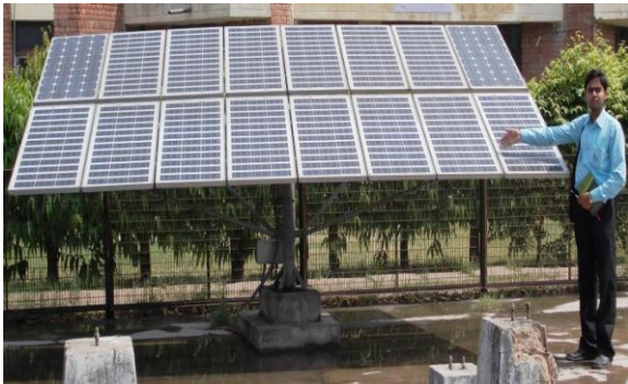
Fig.1- Solar Panel installed at MGICC-Delhi Govt., Alipur-Bakauli, New Delhi
