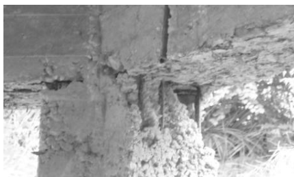
Figure 7 A reinforced concrete beam – column joint with honeycomb
