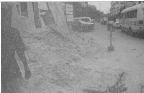
Figure 2 Improper storage of aggregates at a construction site in Dar es Salaam
