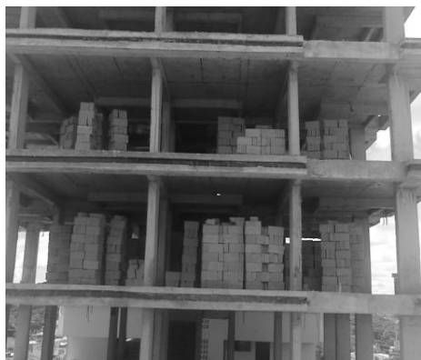
Figure 10 A building frame subjected to premature loading
