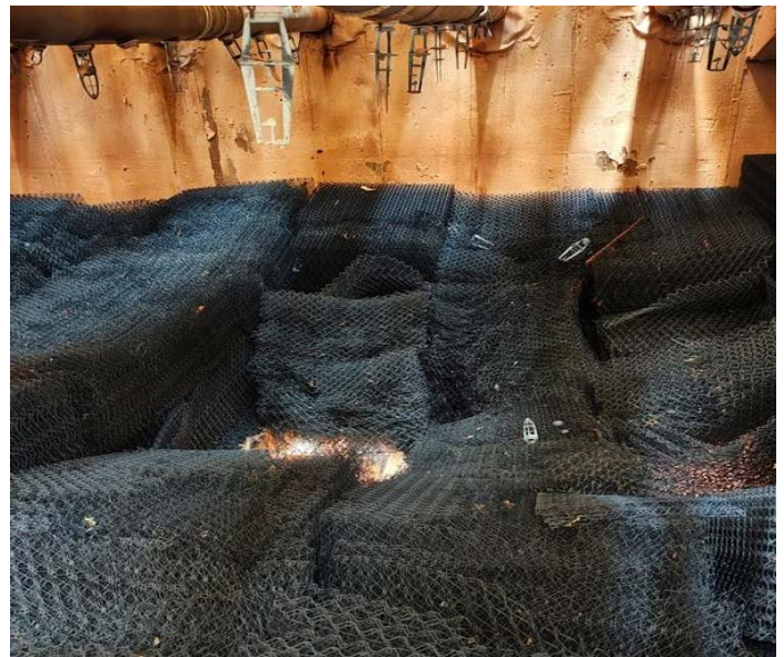
Figure 26: Damaged NDCT fills and nozzles
