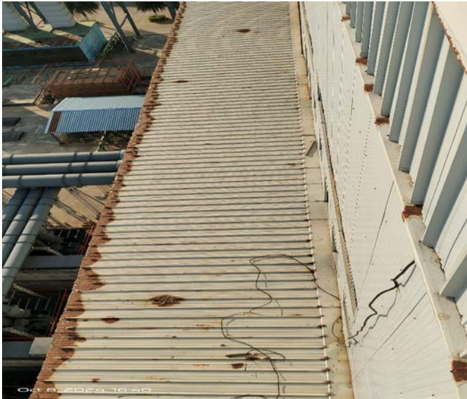
Figure 21: Corroded turbine building sheeting
