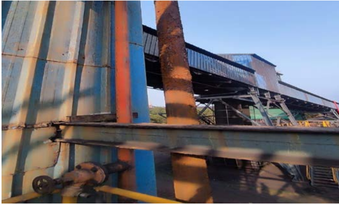
Figure 32: Corrosion on coal conveyor structure
