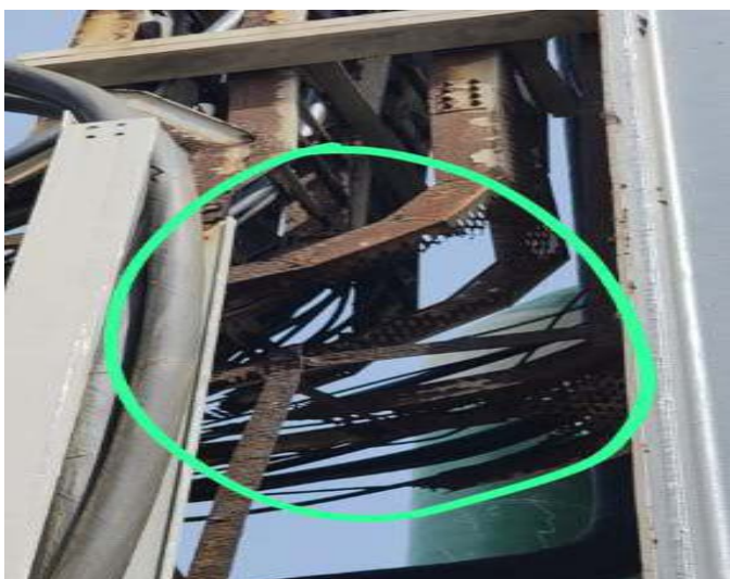
Figure 23: Corroded cable trays
