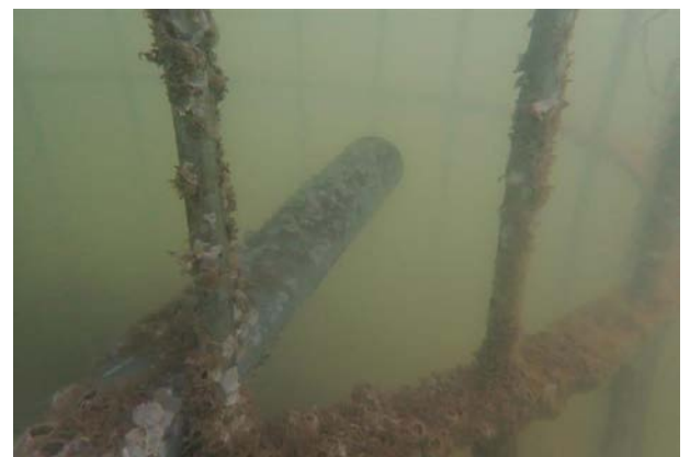
Figure 8: chlorine dosing pipe inside strainer
