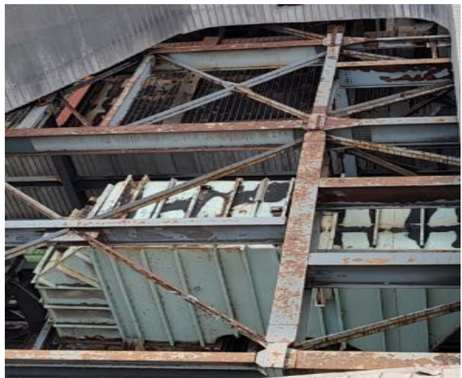
Figure 30: Corrosion on boiler structures
