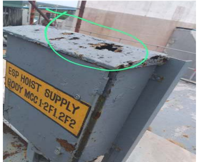
Figure 24: Corroded electrical supply panels
