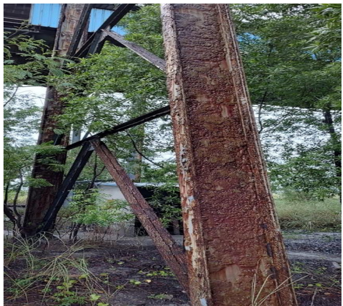
Figure 31: Corrosion on AHP conveyor structure
