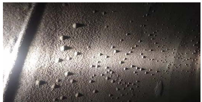
Figure 19: Blisters inside pipeline
