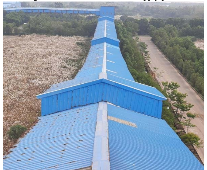
Figure 25 conveyor gallery early stage of corrosion
