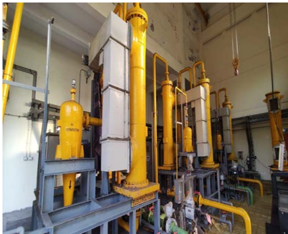
Figure 14 : Electro chlorination plant
