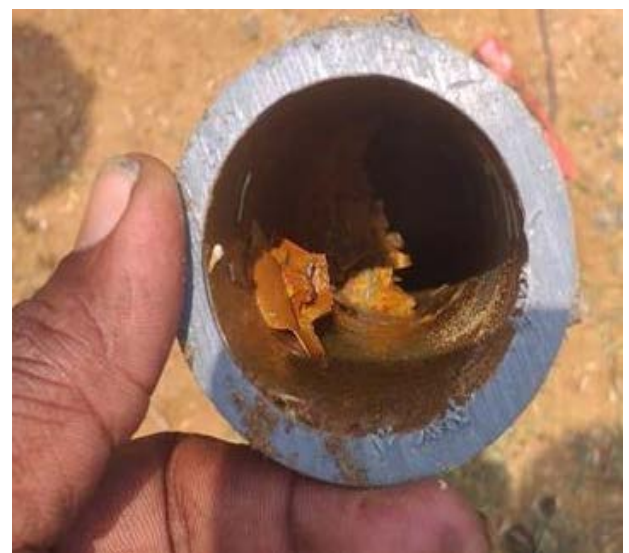
Figure 9: Scaling inside chlorine dosing pipe
