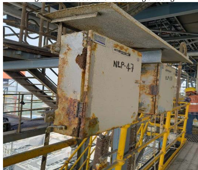
Figure 22: Corroded electrical panels
