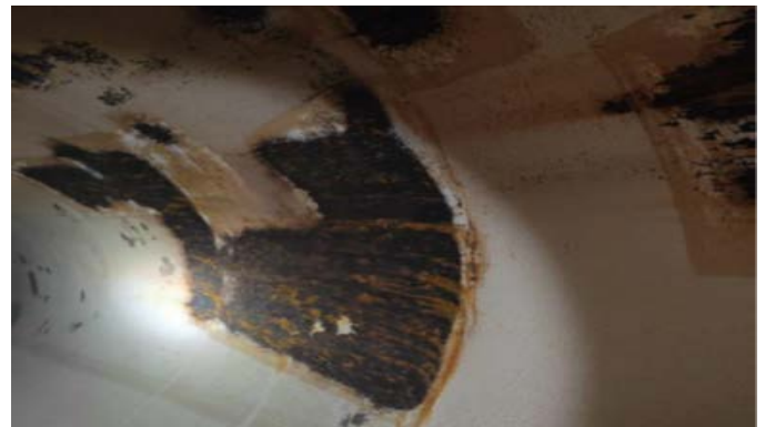
Figure 17: Corrosion in condenser cooling water pipeline
