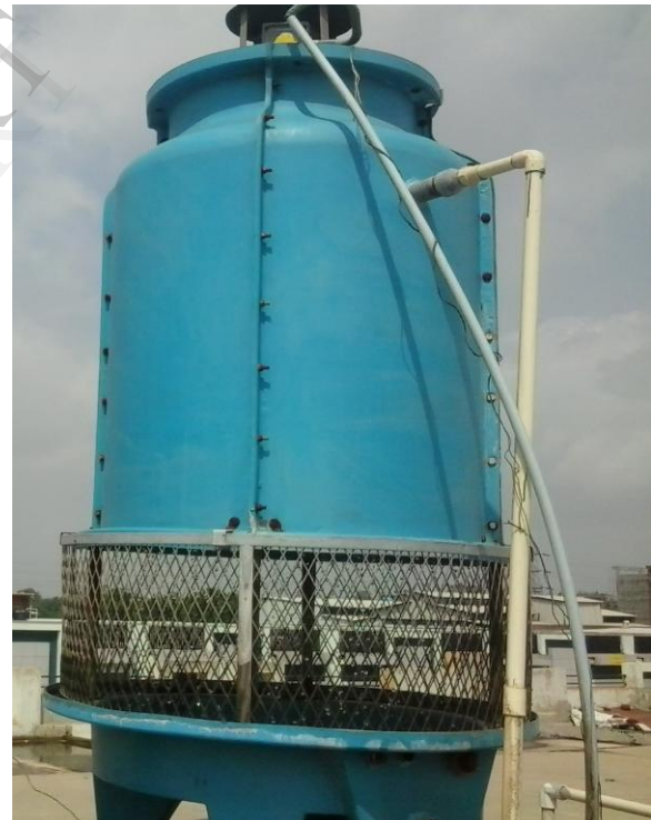
Fig cooling tower for practical reading
