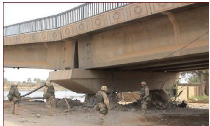
Fig1: A bridge in Iraq damaged by a relatively small number of explosives placed in a Terrorist attack.
