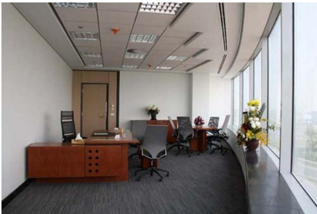
Figure 6. Lighting system in office space. (3).
