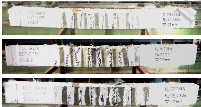
Fig. 9 The cracking pattern of beam STLG
