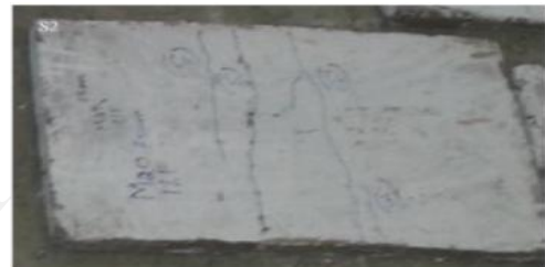
Crack pattern of slab M 20 75mm thickness 1% fiber
