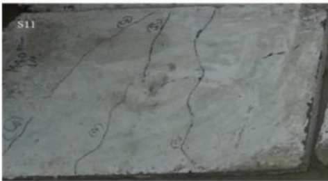
Crack pattern of slab M 40 50mm thickness 1% fiber
