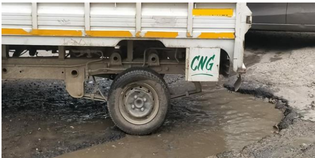
Fig. 1. Image description of potholes in an unstructured environment
