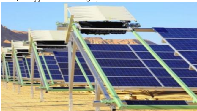
Fig. 2. Ecoppia E4 Cleaning System
