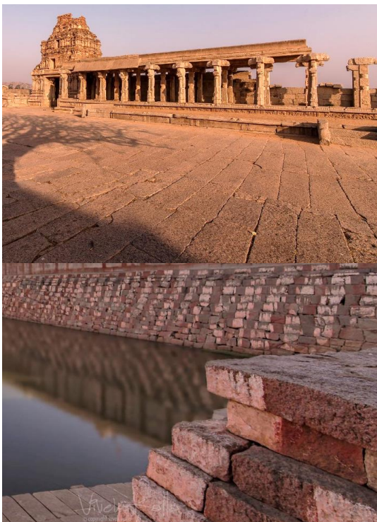
Photos depicting the ancient stones in its dilapidating state which needs utmost care while executing repair works.
