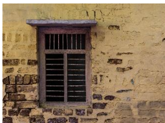
Photos showing under maintained brick wall getting weathered due to direct exposure of weather conditions.
