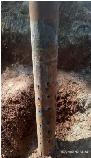
Fig 4: Holes on casing pipe.
