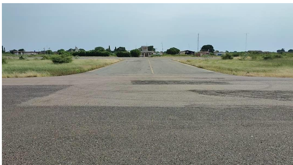
Figure 2: erosion in apron area
