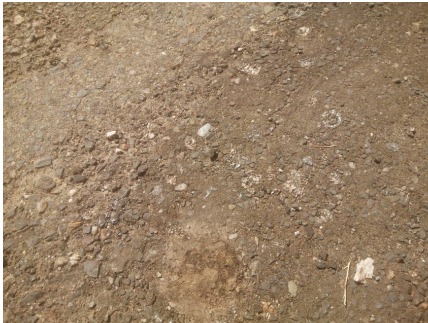
Figure 1: surface layer erosion of runway pavement
