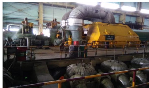
Fig-2 Power plant view
