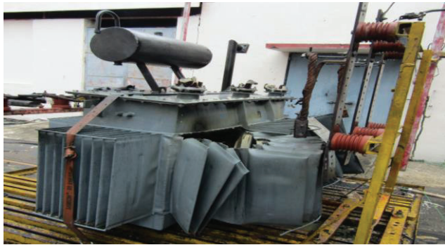
Fig 4. Distortion on HV side of 400 kVA, Transformer
