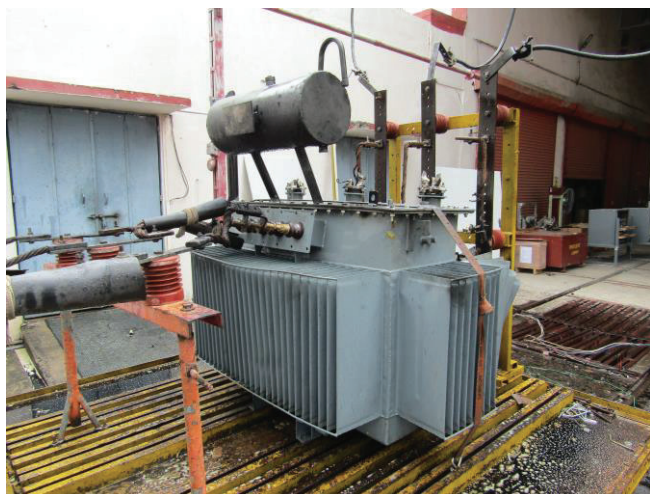
Figure 5. Distortion on LV side of 400 kVA, Transformer
