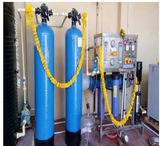
Fig.7. Photograph of hardware setup of water purification plant
