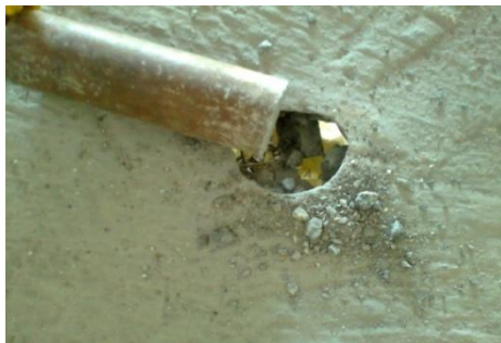
Fig 9 Ultimate failure on specimen
