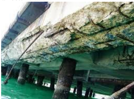
Fig. 1 Bridge Subjected To Chloride Attack
