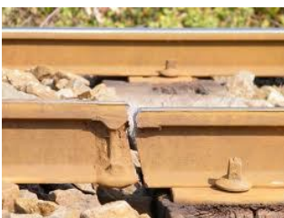
Figure.1 Railway Track Defect
