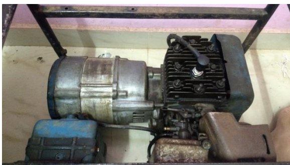
Fig 5: engine connected to alternator
