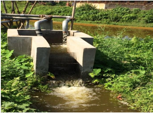
Fig 4: The collecting chamber that receives the water from the pump
