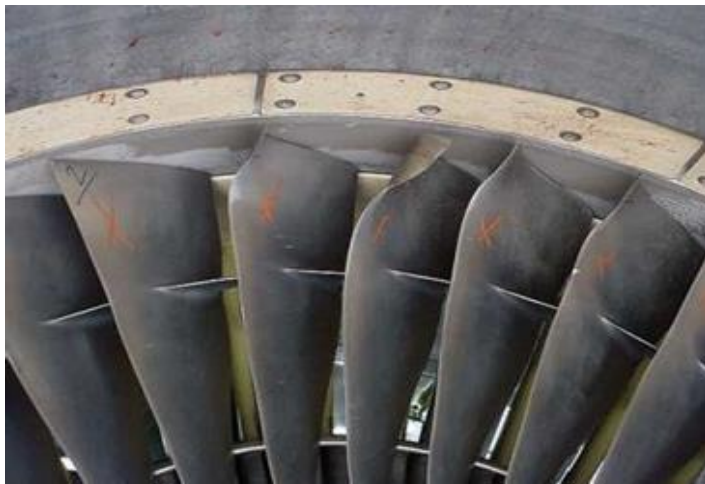
FIG 2.4.1.2 ENGINE BLADE DAMAGE DUE TO AN INGESTION OF A SMALL BIRD
