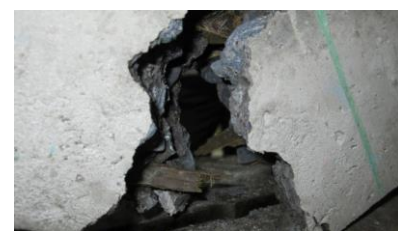
Fig.13: Failure of Doubly Reinforced Beam
