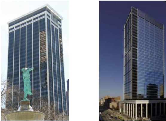
Figure 4: (a) One Indiana Square tornado induced damage (b) Remodeled façade of building
