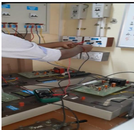
Fig 3.6 Solar power control
