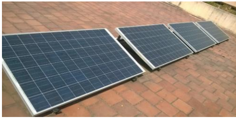
Fig 3.4 Solar Panel (250W*4=1000W)
