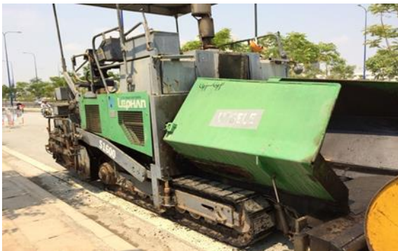
Figure 14. Application of RCC spreader for road works, similar to hot asphalt concrete carpeting
