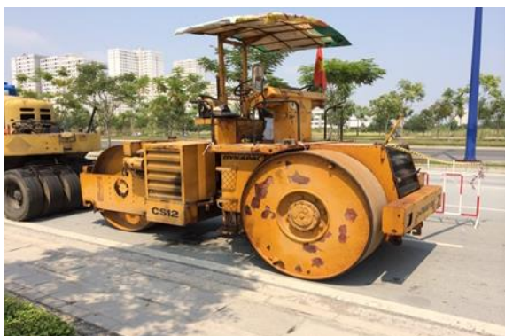
Figure 16. Application of iron wheel roller to smooth RCC surface for road works, similar to hot asphalt concrete
