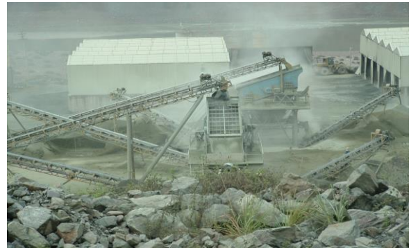
Figure 2. Stone aggregate crushing and screening station of all sizes according to the correct gradation
