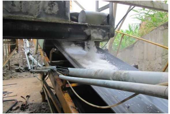
Figure 9. Portion of the water feeding to the RCC mixture is cooled to ice
