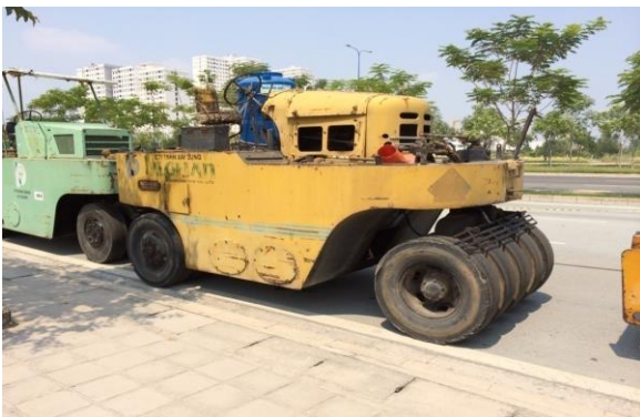
Figure 15. Application of rubber wheel roller to smooth RCC surface for road works, similar to hot asphalt concrete
