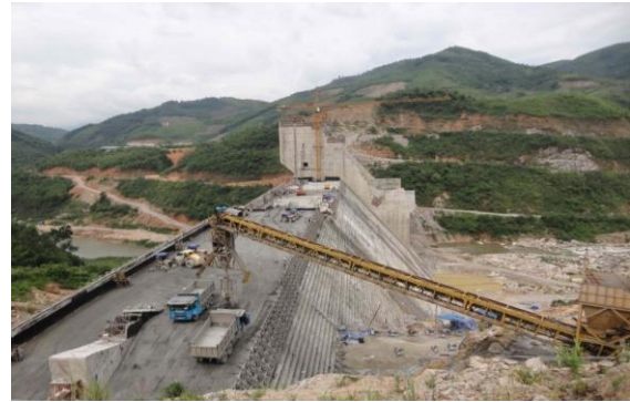
Figure 1. RCC equipment line: Mixing RCC mixture at the station, transporting to the field by conveyor and dump truck, leveling and compacting
