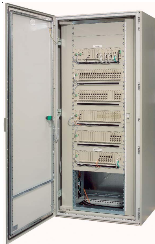
Fig 3: ABB RTU560A Panel at 110/11 kV substation [5].
