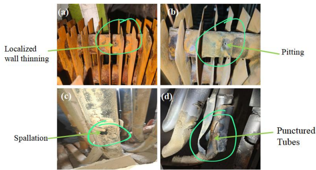
Fig.1 Damage and perforation of the boiler tubes were caused by erosion-corrosion (TSPCL)
