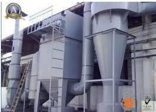
Fig 3 Dust Collector System
