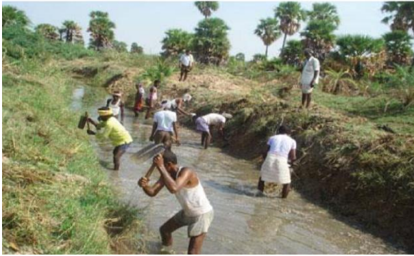
Fig 1: Channel System Irrigation
