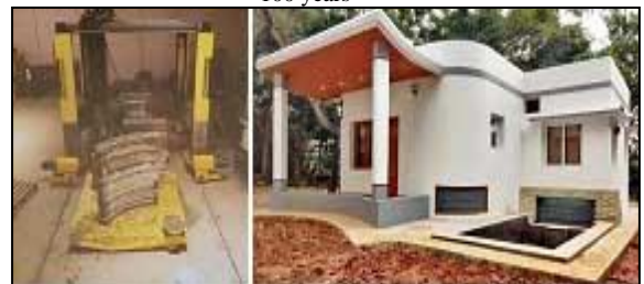
Fig -5: India’s first Industrial size 3d Concrete printer at IIT Madras by TVASTA & India’s first 3D Printed house at IIT Madras (3DParts printed by Offsite printer, transported and assembled at site.)
