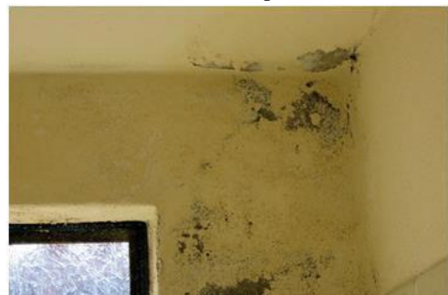
Fig.1. Image showing damages occurred in roof and wall due to water leakage
