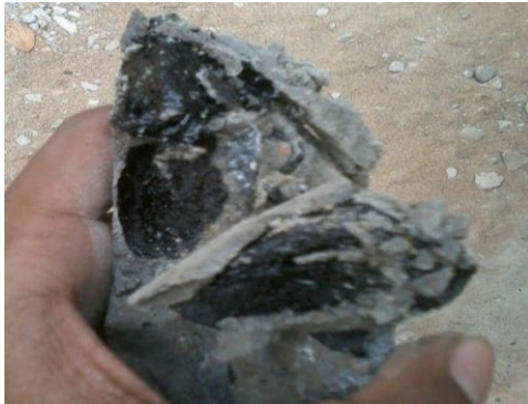
Fig 11 BCA in Concrete After Failure
